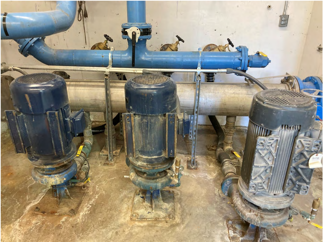
Figure 34 - Pumps at Impure pump Building
