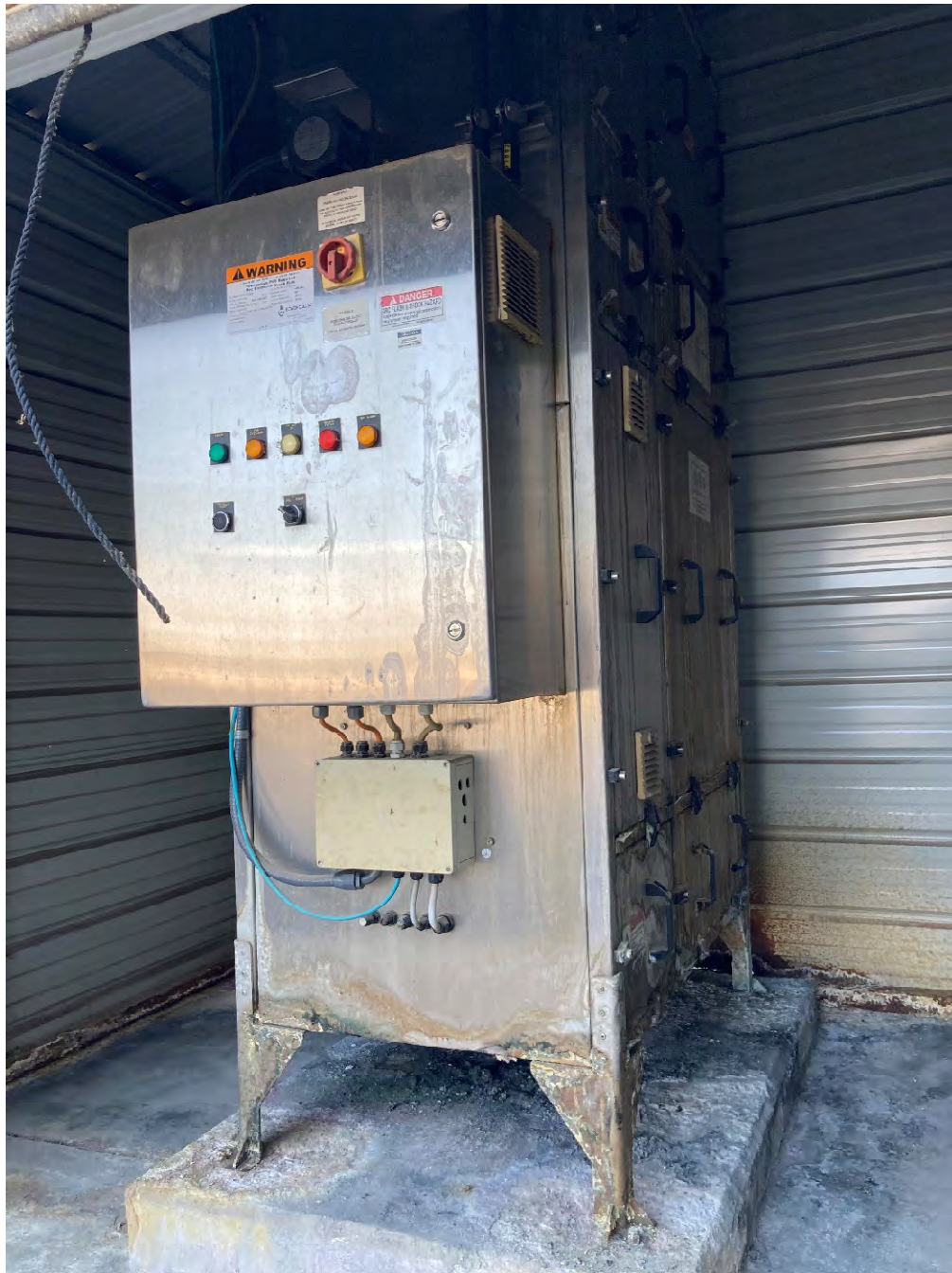
Figure 25 – Odor Control unit at Thermophilic Digester
