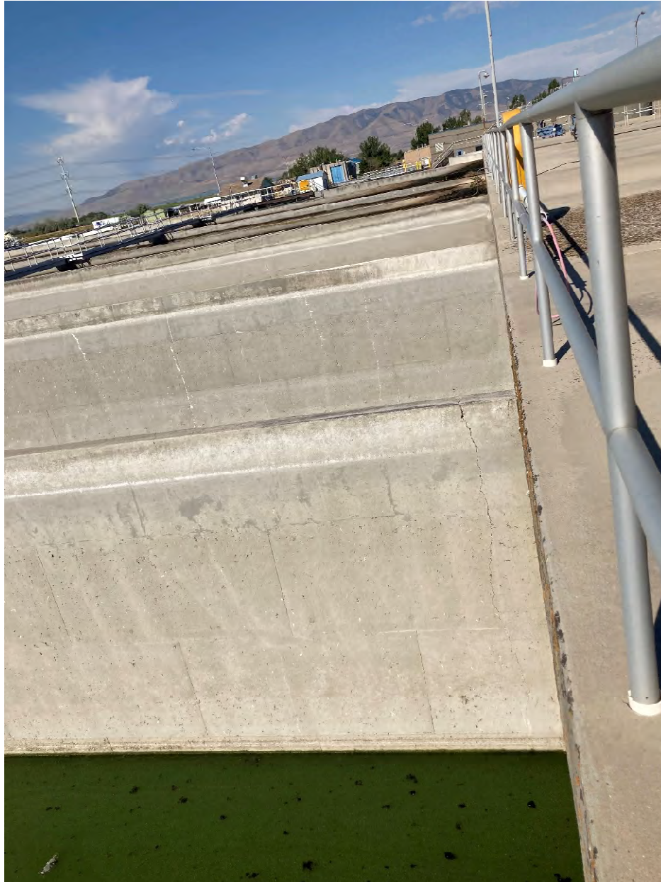
Figure 15 – Spalling of concrete and cracks on Bioreactor No. 2 walls
