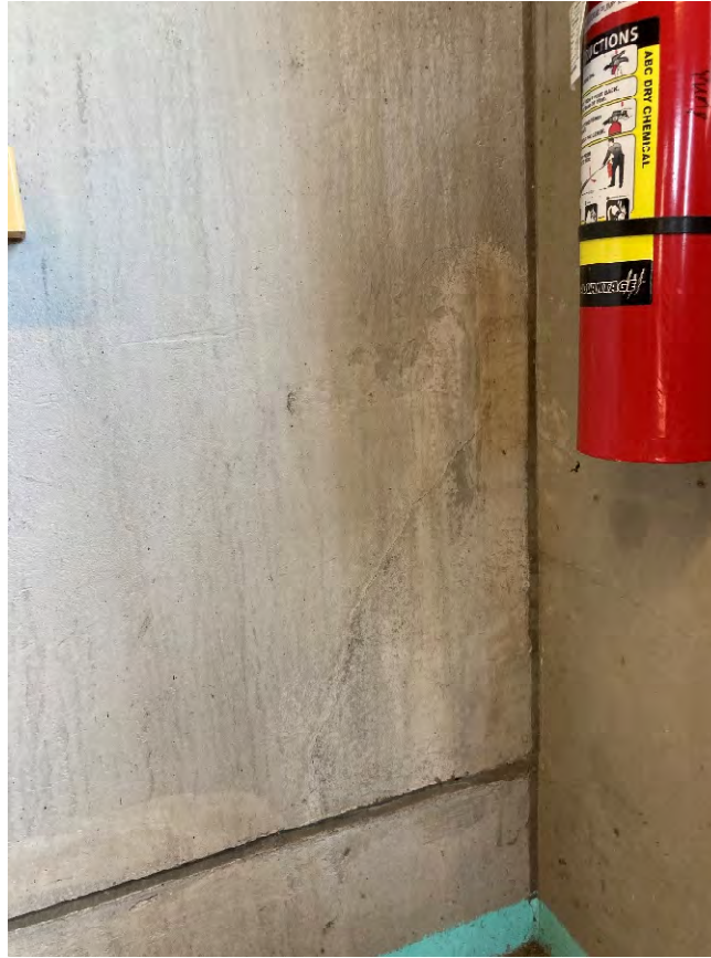
Figure 10 - Cracks inside the Primary Sludge Pump Building
