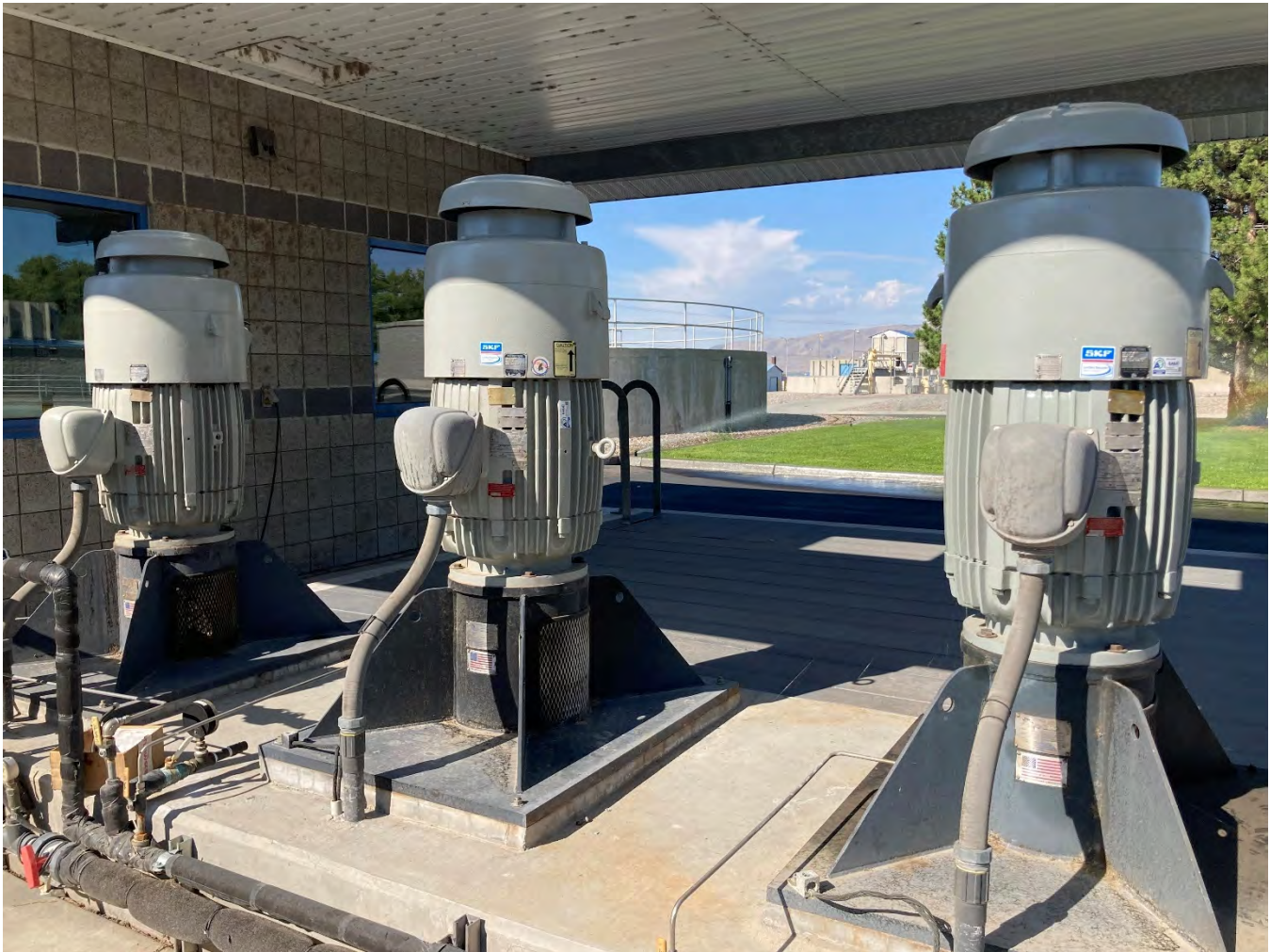
Figure 12 - Mixed Flow Pump Station
