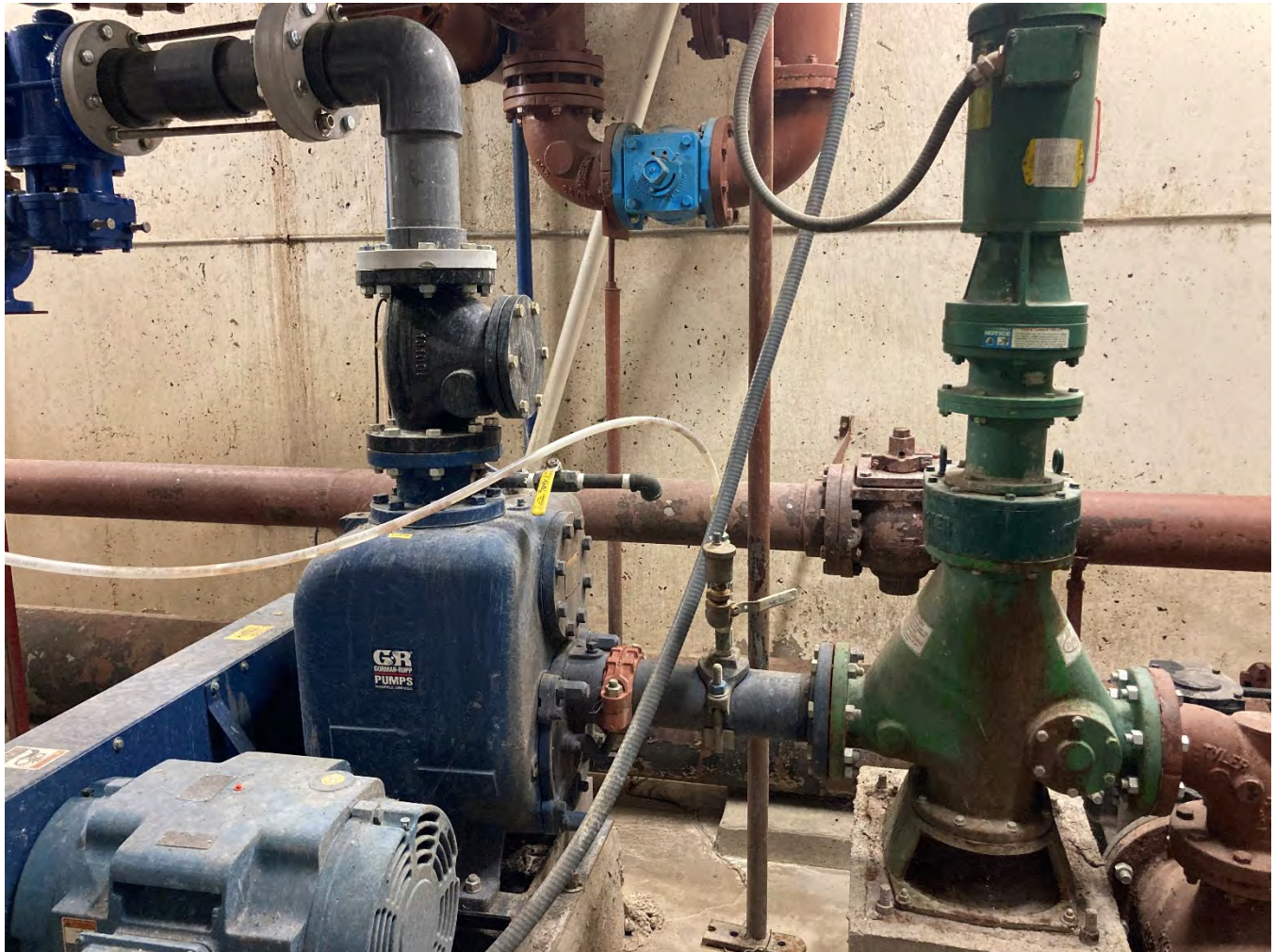
Figure 28 – Grinder pumps at Aerobic Digester Building
