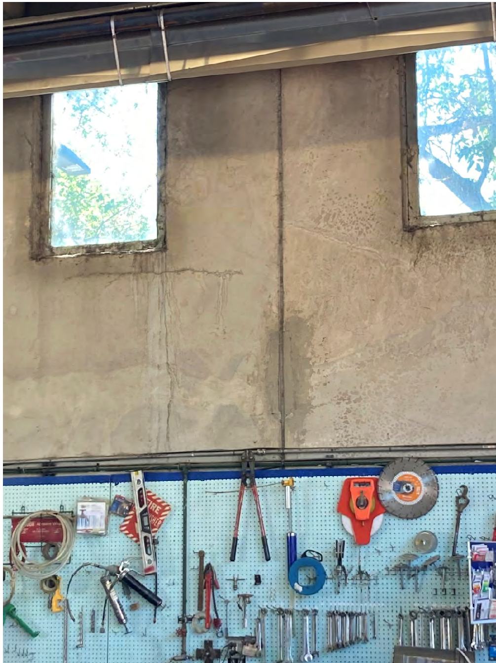
Figure 33 – Deterioration at Maintenance Shop Building
