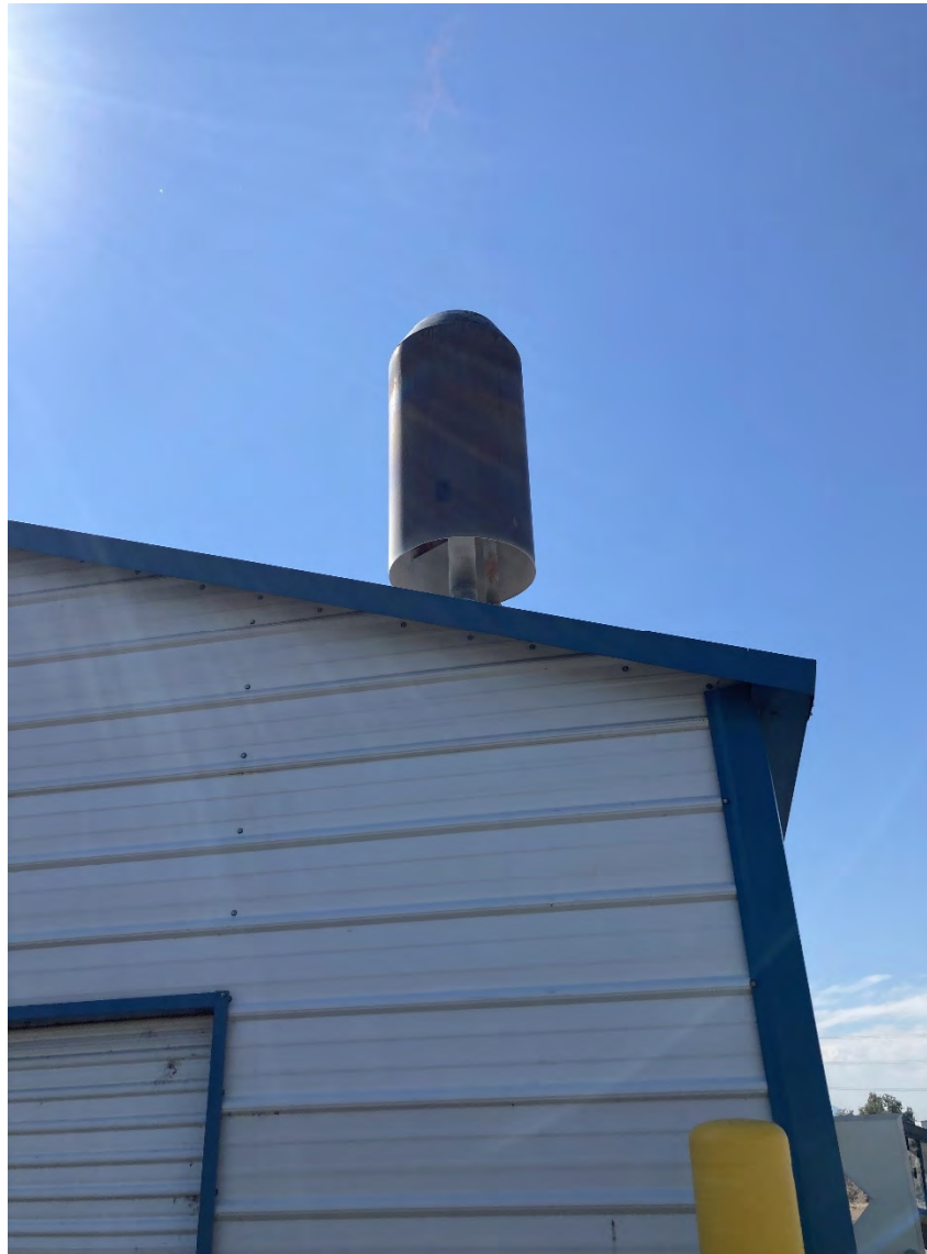
Figure 32 – Flare stack near Thermophilic Digester
