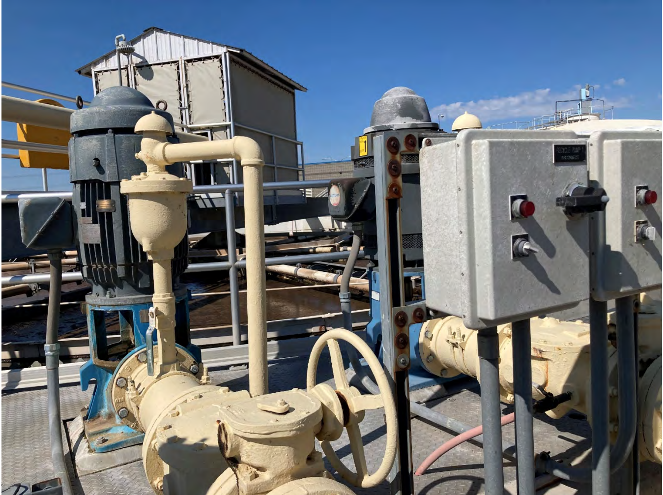
Figure 23 – Electrical disconnects and recycle pumps at the DAF
