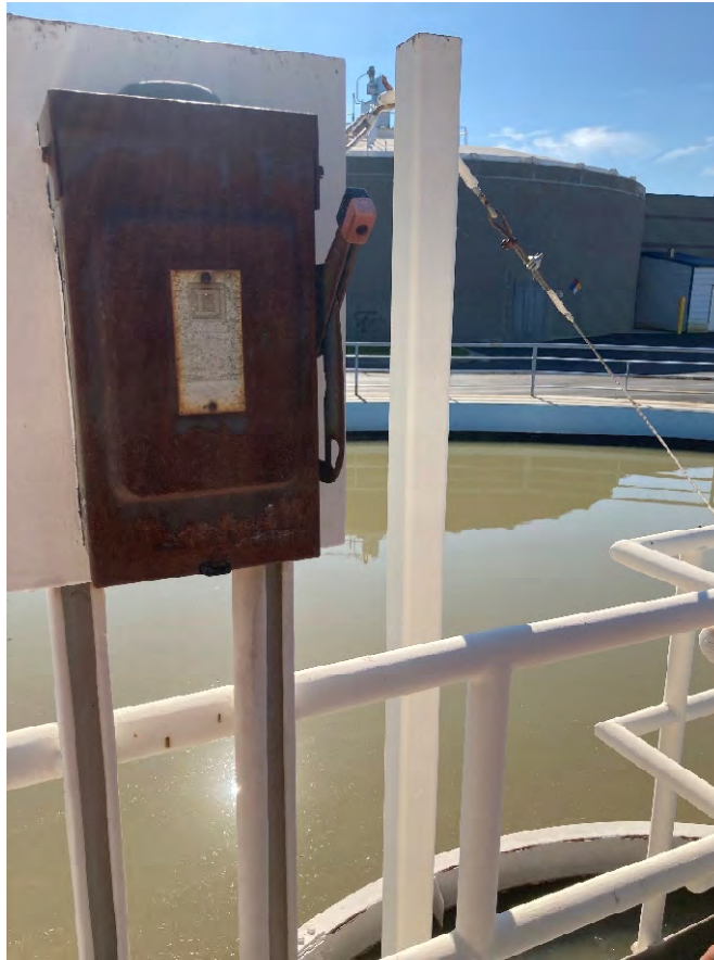
Figure 8 - Electrical disconnect at the Primary Clarifiers
