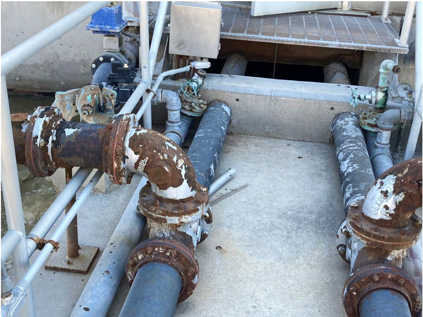
Figure 7 - Worn out and leaking air piping at Aerated Grit
