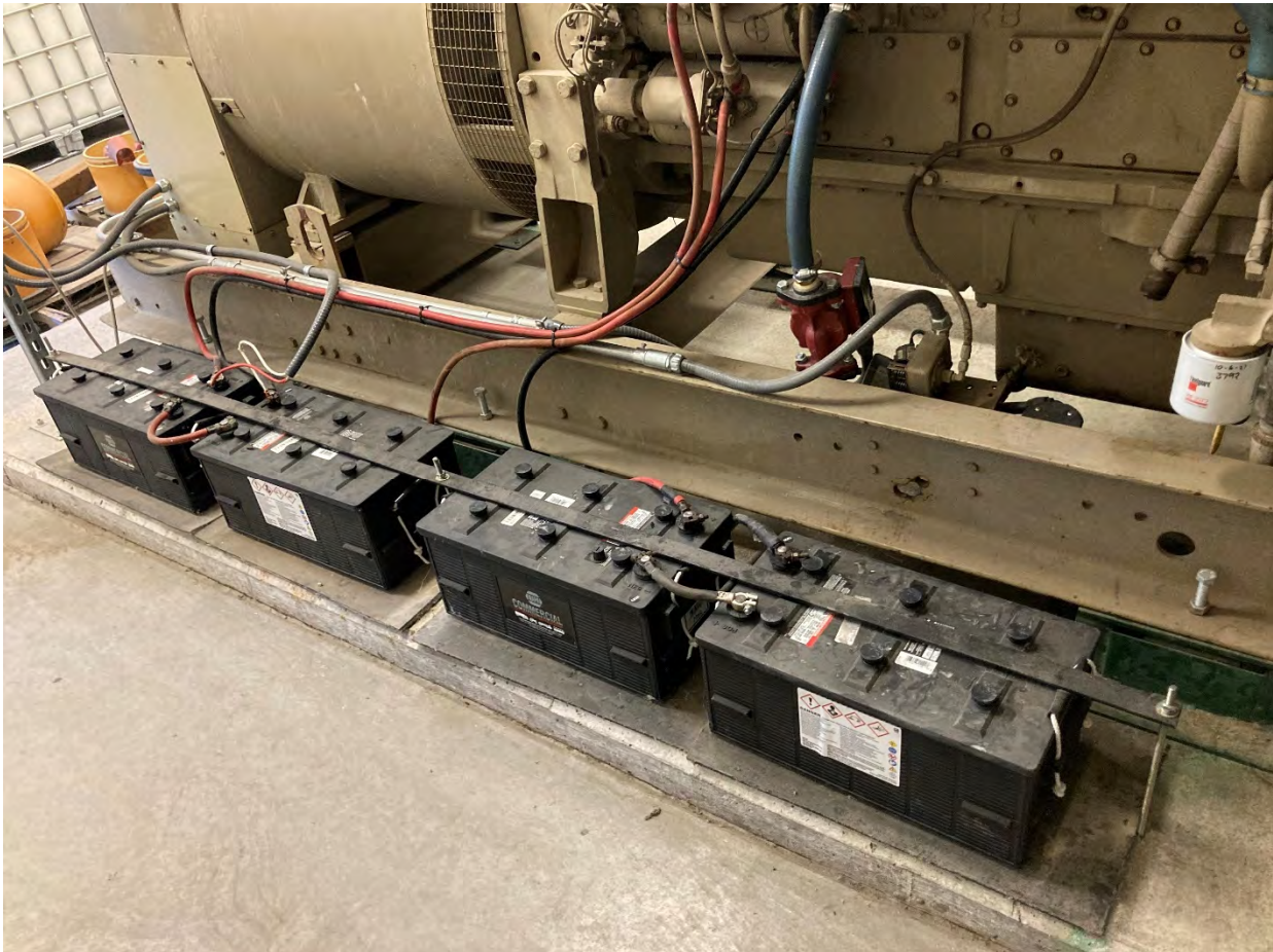
Figure 18 - Generator batteries at Bioreactor Blower Building
