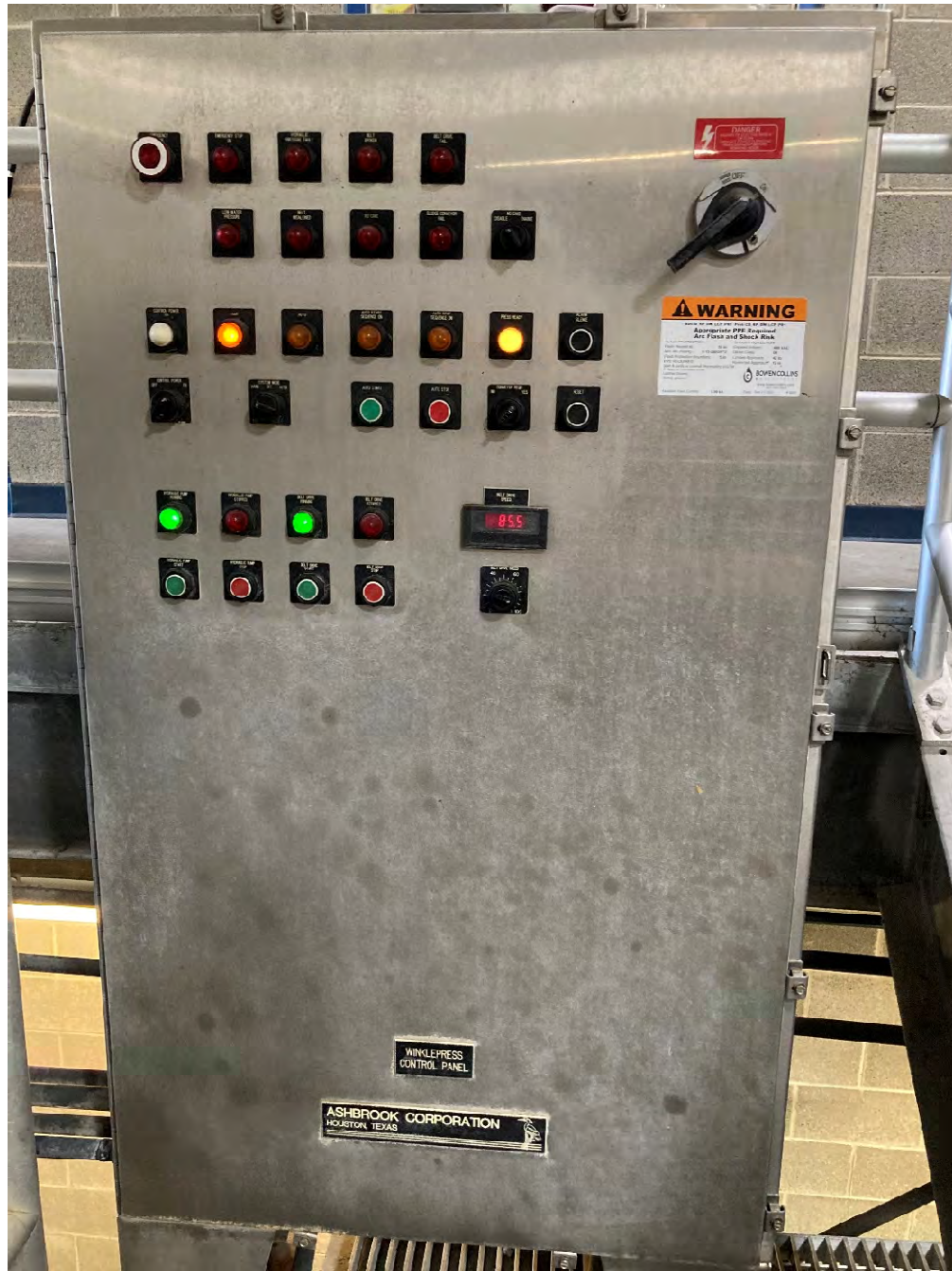
Figure 31 - Belt Press control panel
