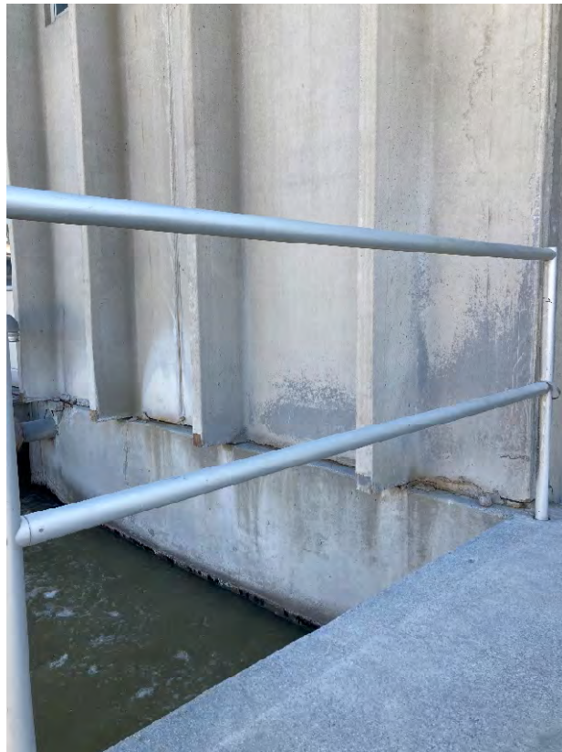
Figure 5 – Condition of Headworks Building wall near Aerated Grit Channel
