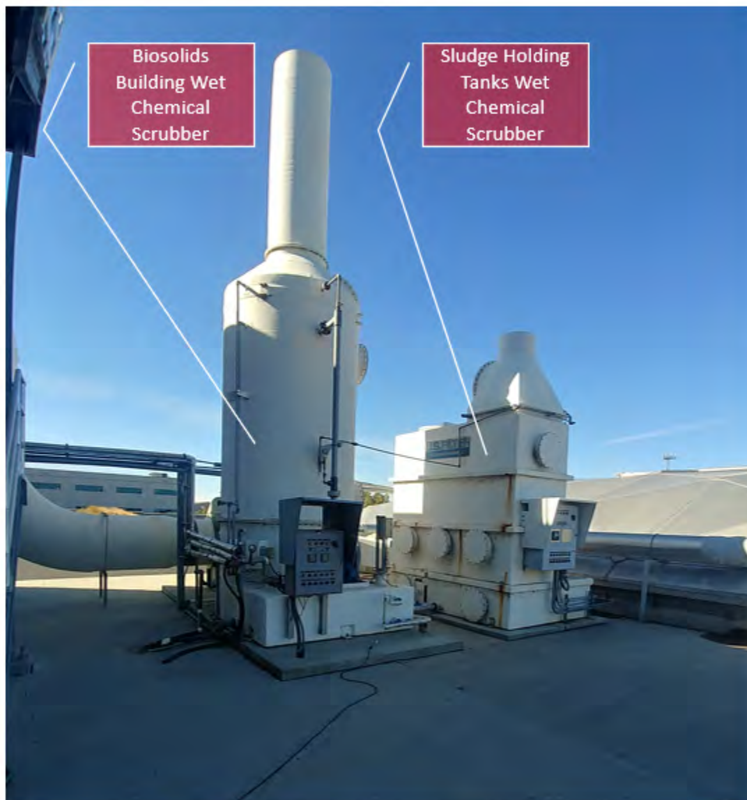
Figure 9: Chemical Scrubber unit for sludge holding tanks (right) and dewatering building (left)
