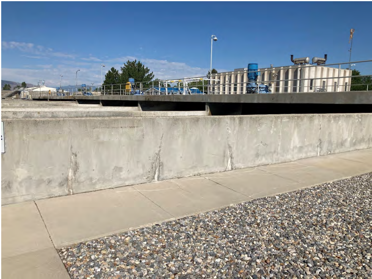
Figure 14 – Bioreactor No. 2 Cracks
