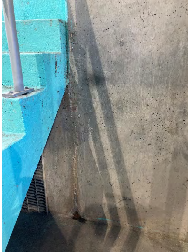
Figure 9 – Cracks inside the Primary Sludge Pump Building
