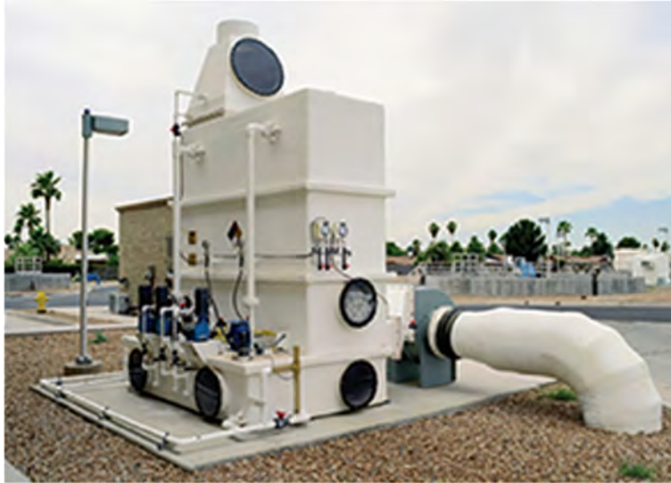
Figure 11: Typical Low-Profile Wet Chemical Scrubber for Odorous Air Treatment
