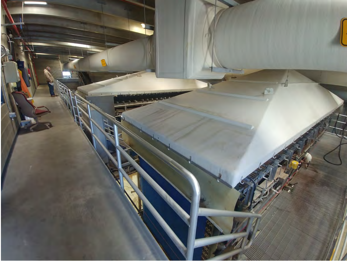
Figure 10: Odor collection hoods over dewatering equipment in Biosolids Building
