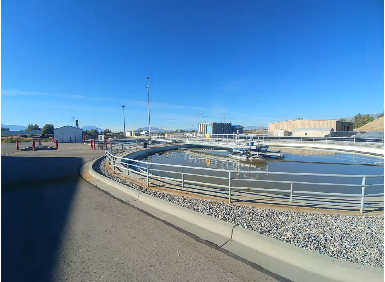
Figure 6: Primary clarifier open to the atmosphere
