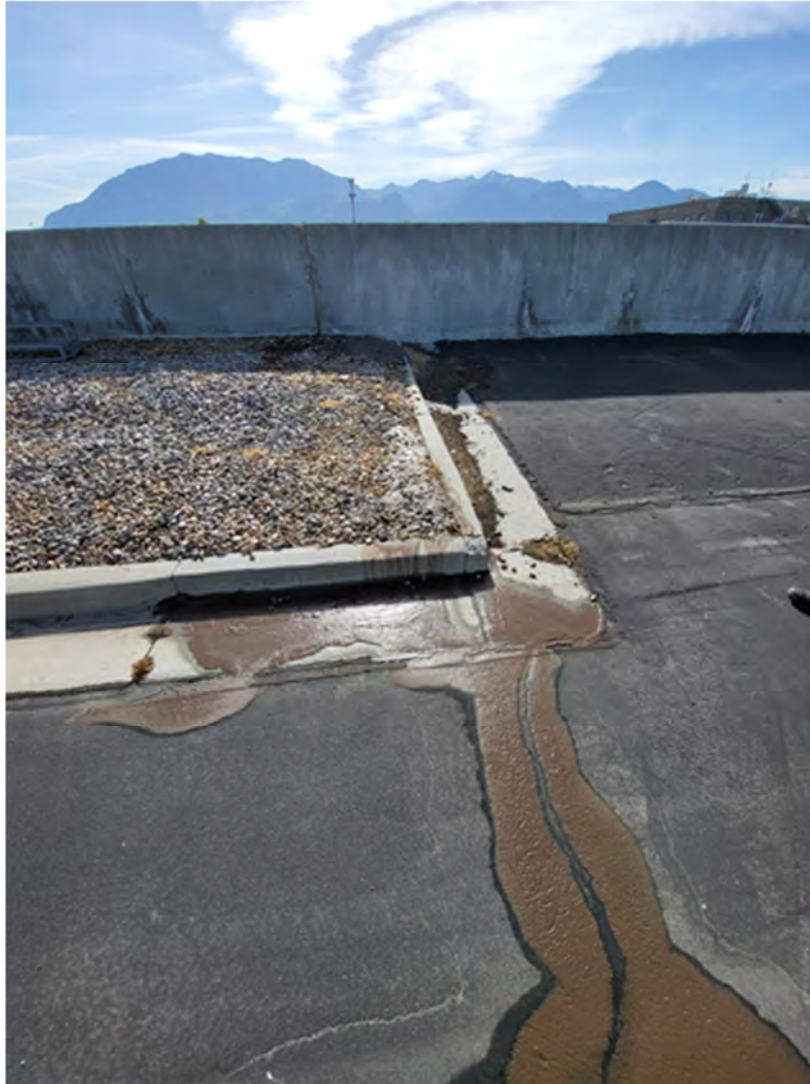
Figure 16 – Sludge on pavement near Bioreactor No.1
