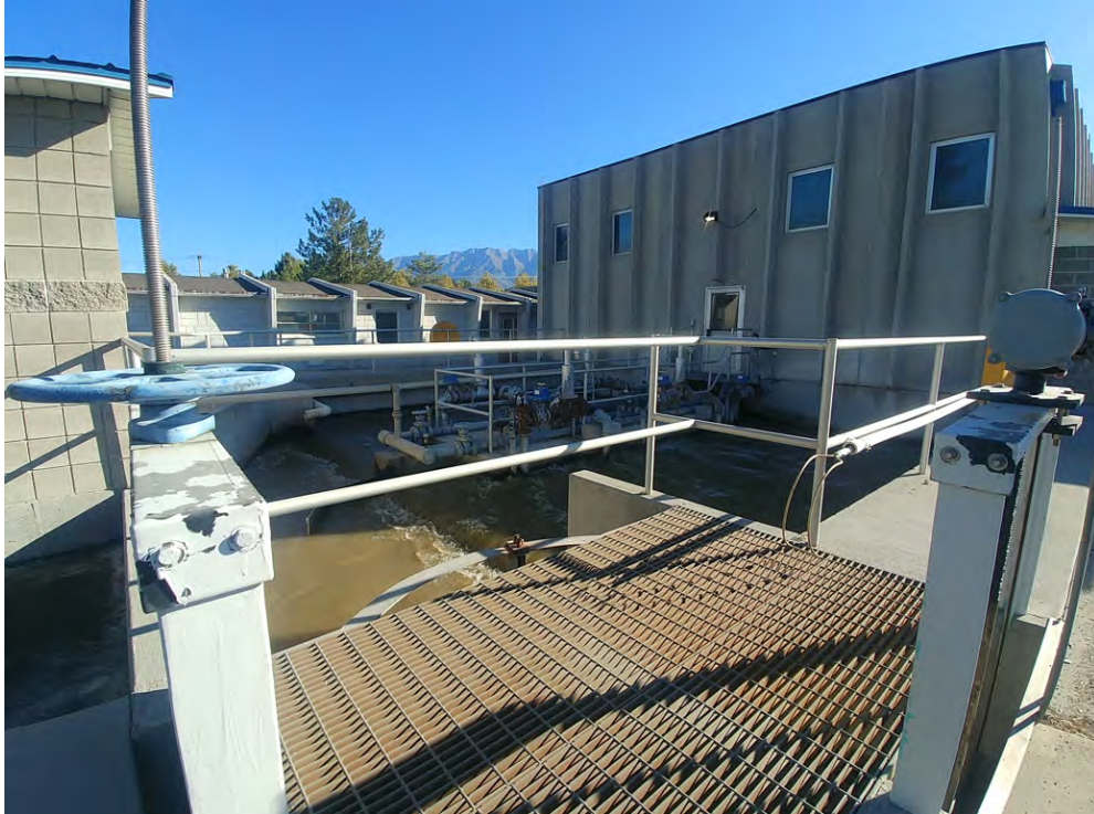
Figure 5: Aerated grit unit open to the atmosphere
