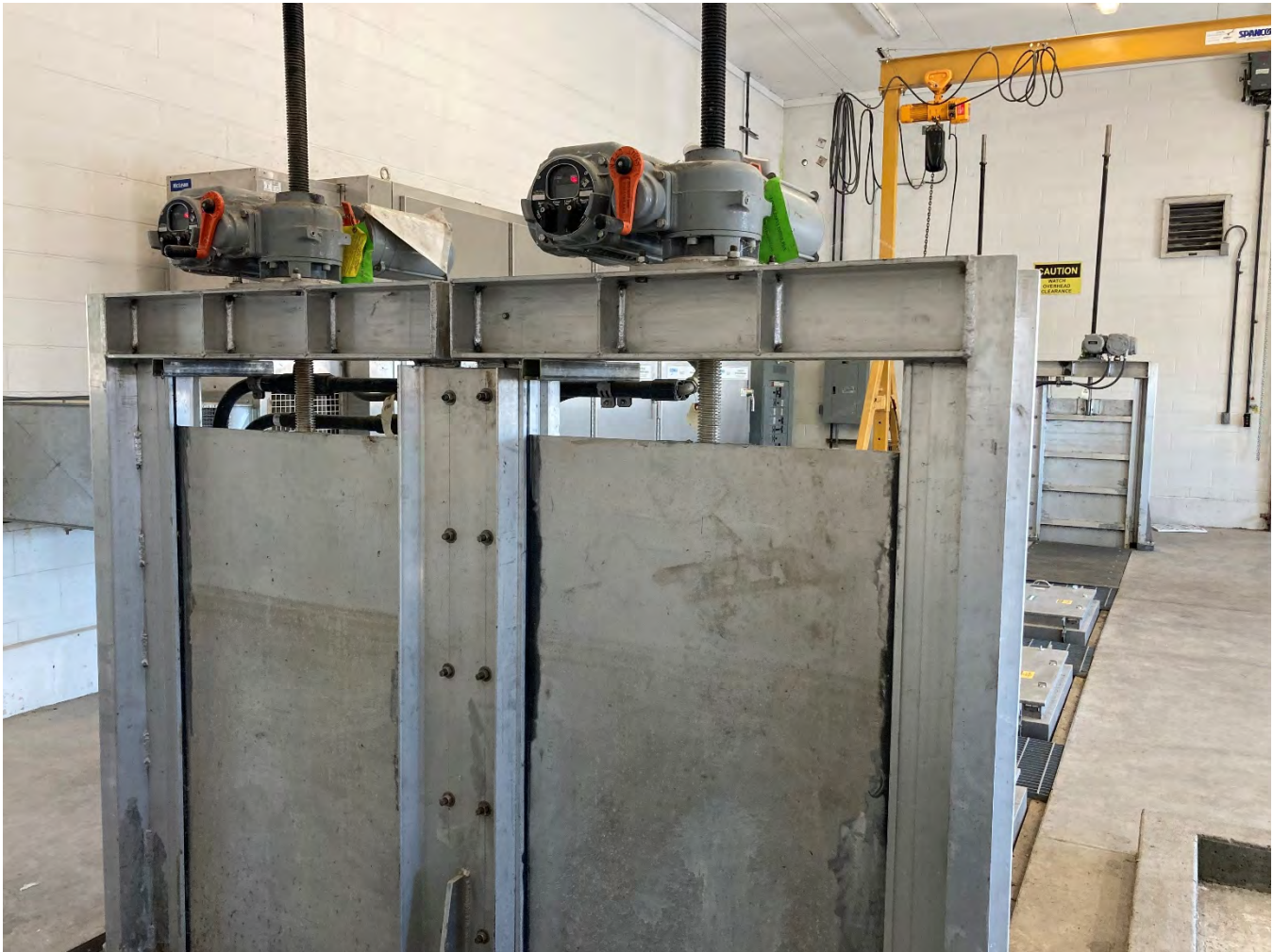
Figure 21 – UV Channel influent and effluent gates with actuators.
