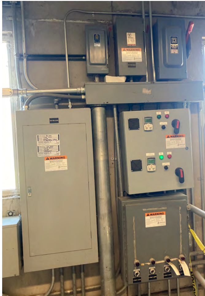
Figure 11 - VFD panel, electrical disconnect at Primary Sludge Pump Building
