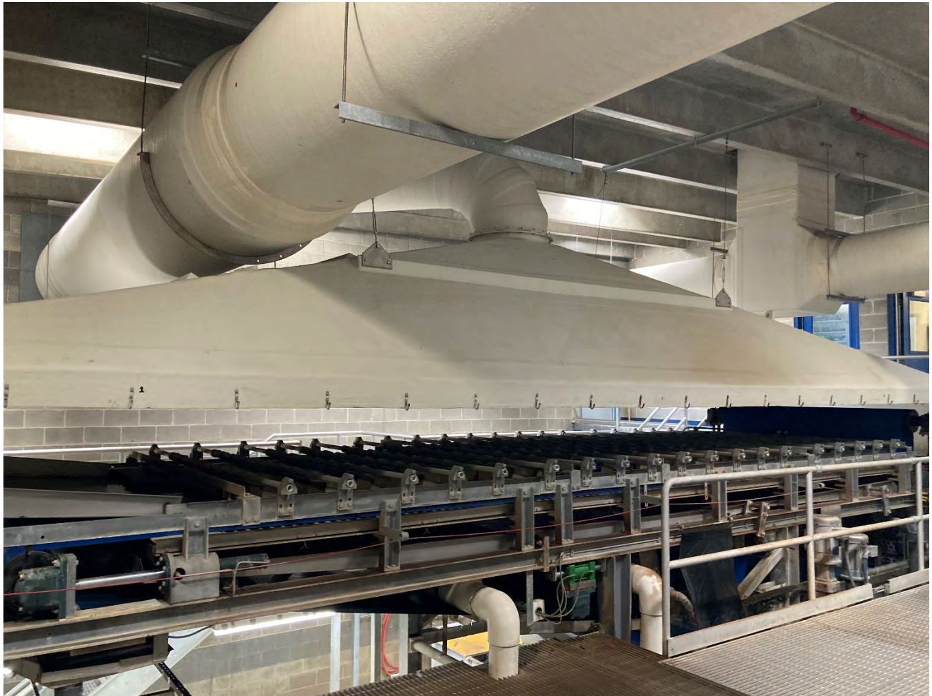
Figure 30 – Belt Press and cover at Biosolids Building
