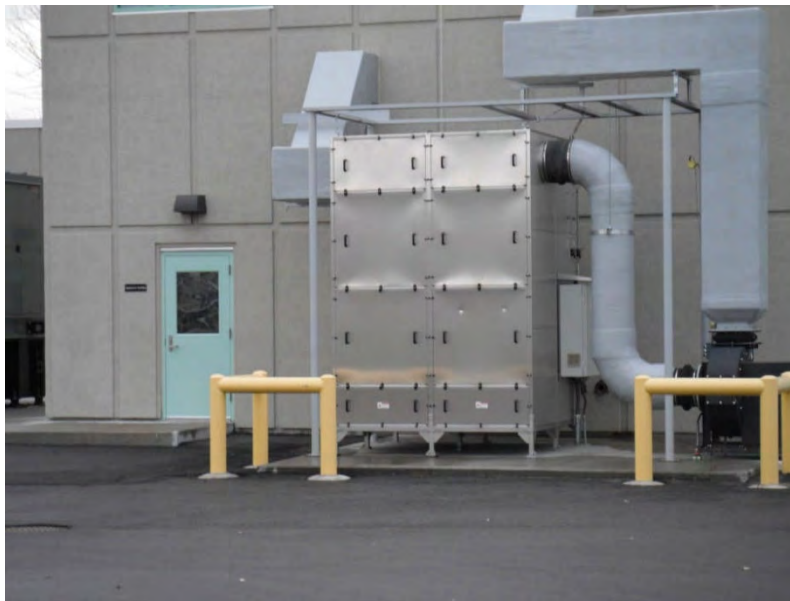
Figure 16: Photoionization Unit Treating Headworks Building Odors
