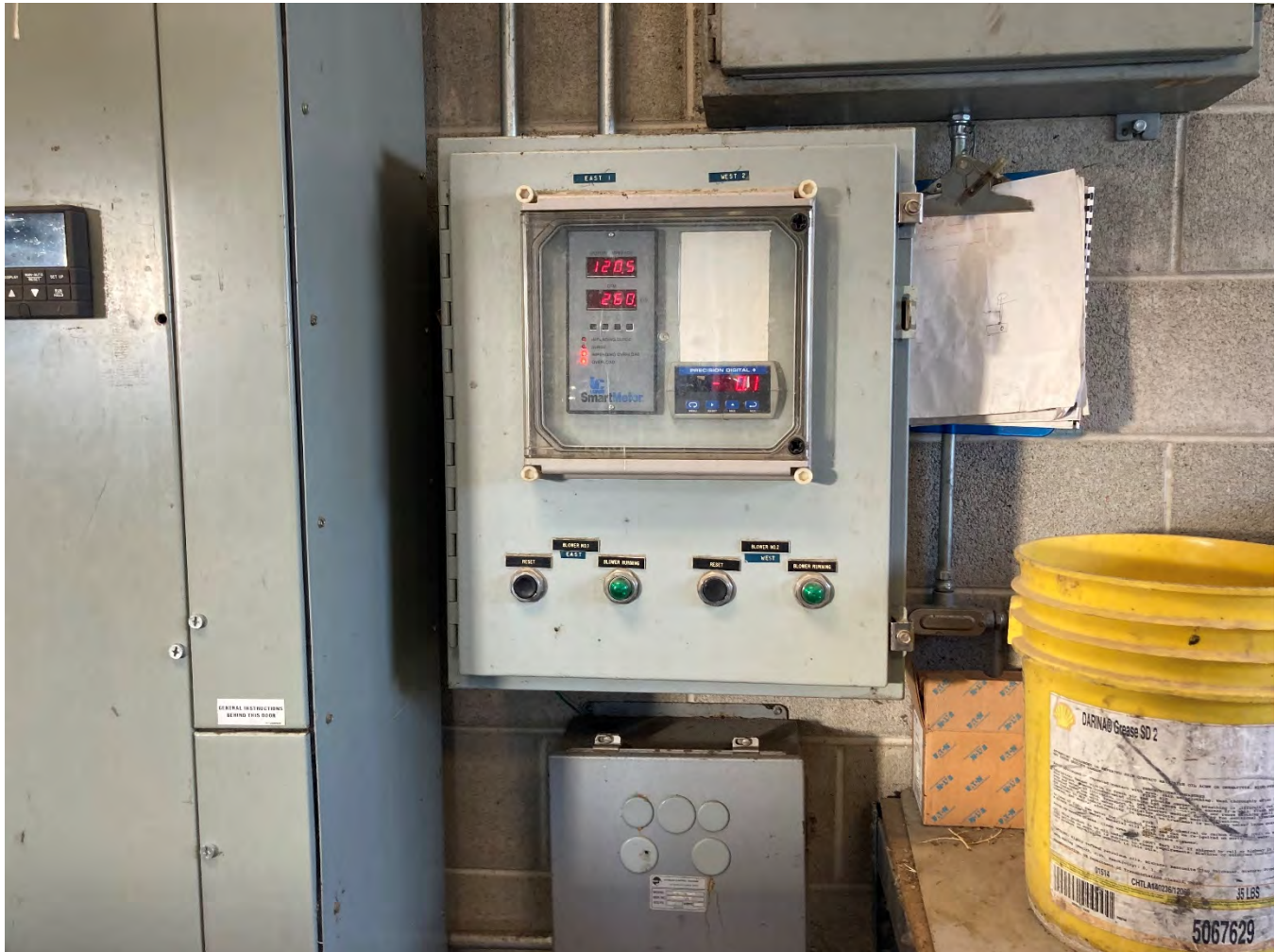
Figure 29 - Blower control panel at Aerobic Digester Building
