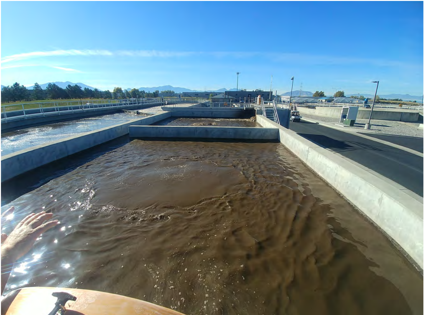
Figure 7: Anaerobic basins with cannon air mixer
