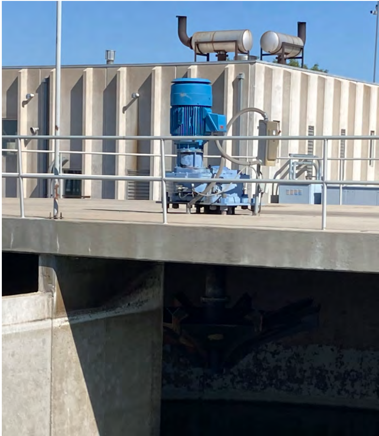
Figure 17 – Surface aerator in Bioreactor No. 2
