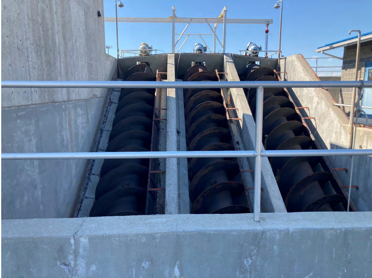
Figure 13 – Screw Pump Station
