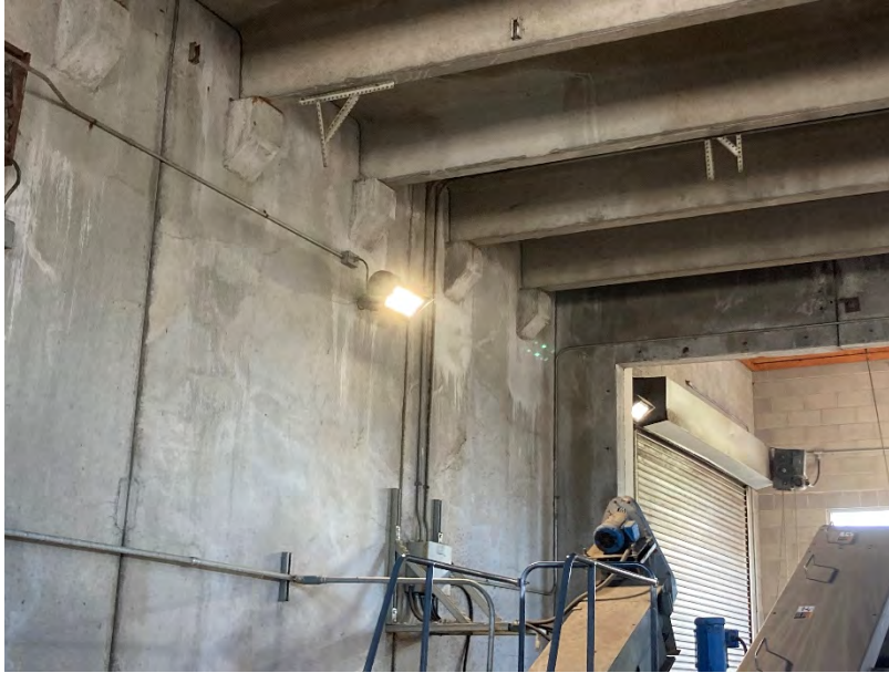
Figure 4 – Spalling of concrete at the beam, cracks on walls, discoloration on walls due to seepage of water through cracks at Headworks Building
