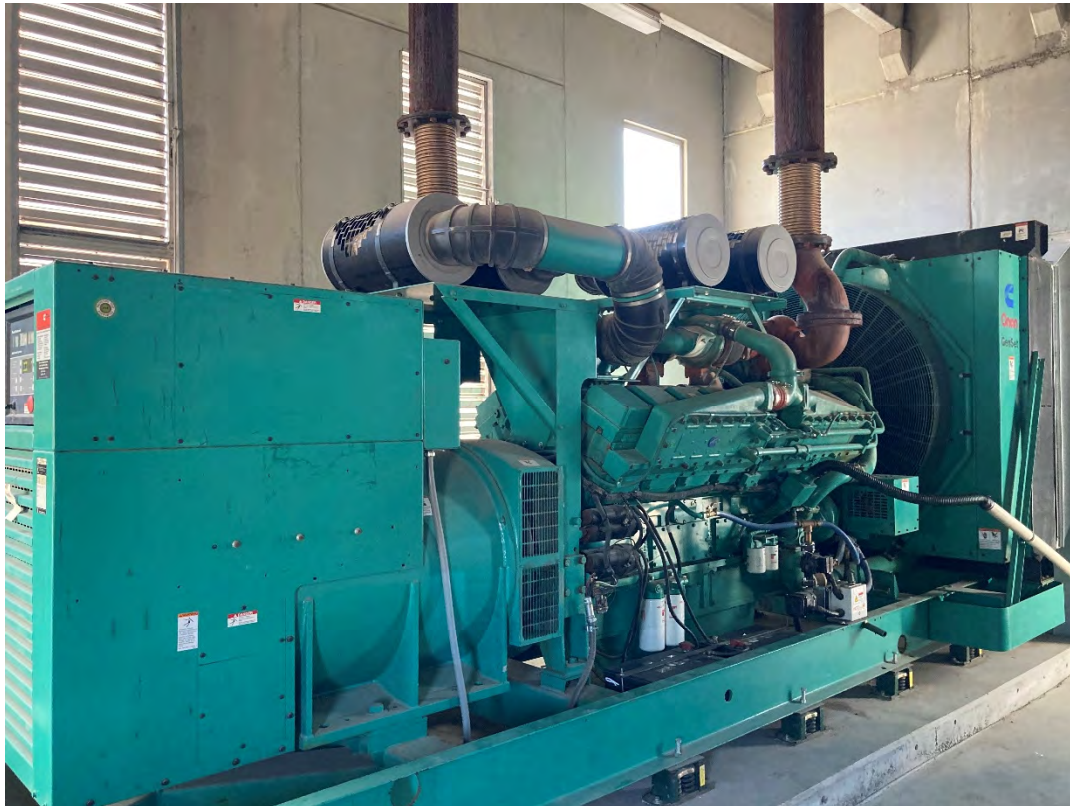
Figure 20 – Generator showing the exhaust system
