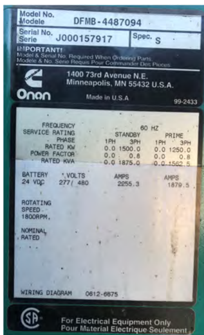
Figure 7-1 – Service 1 Generator Nameplate
