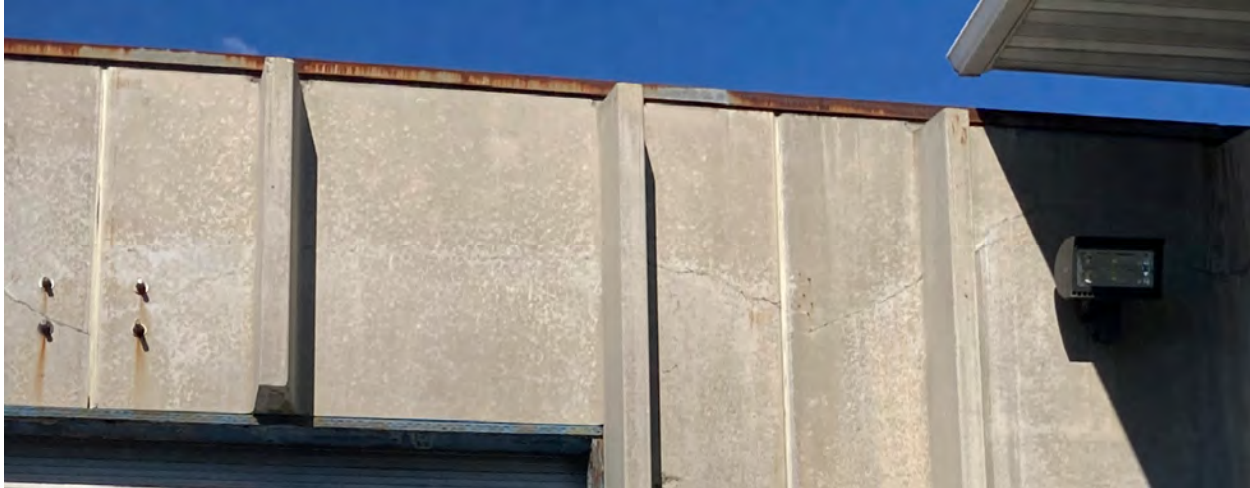
Figure 6 – Cracks on Headworks Building near overhead door
