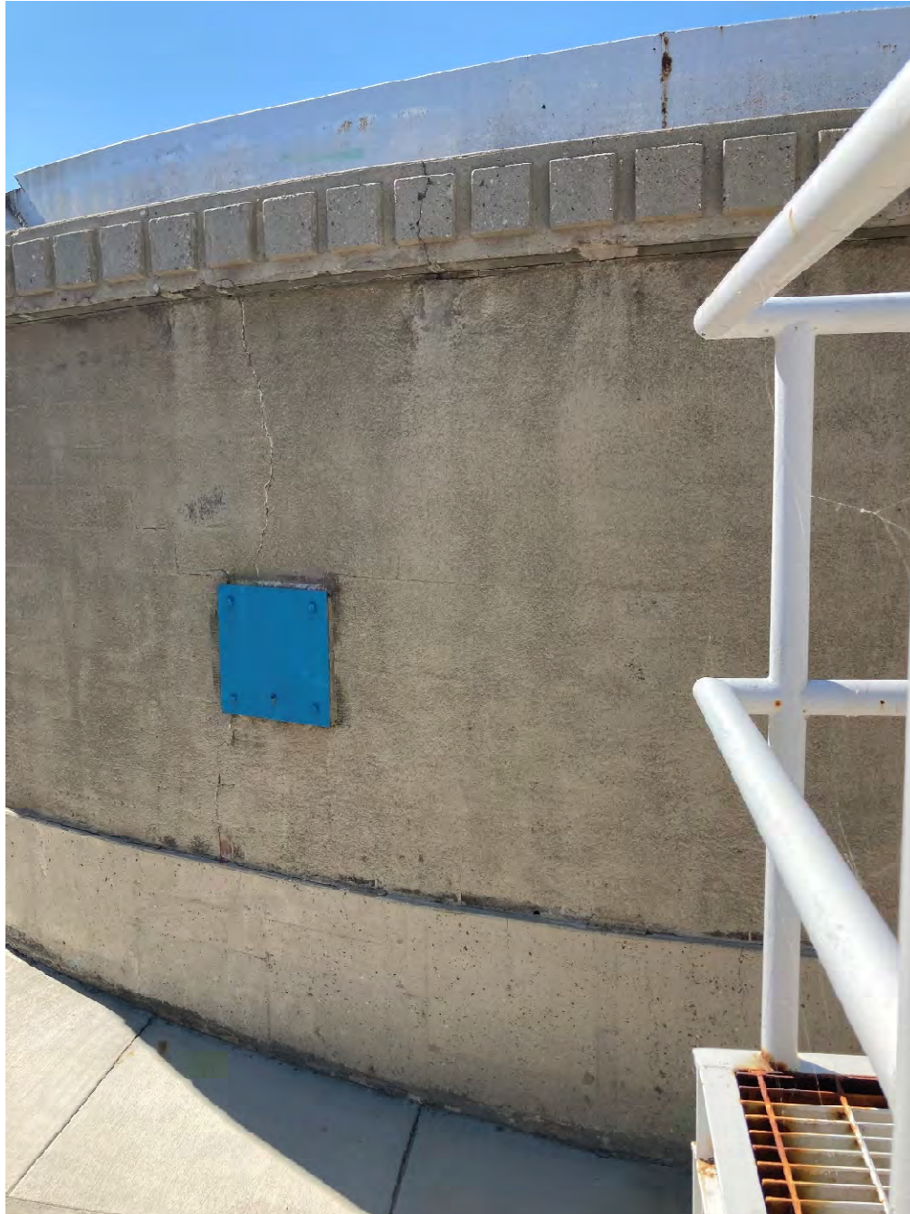
Figure 27 - Cracks on mesophilic digester tank
