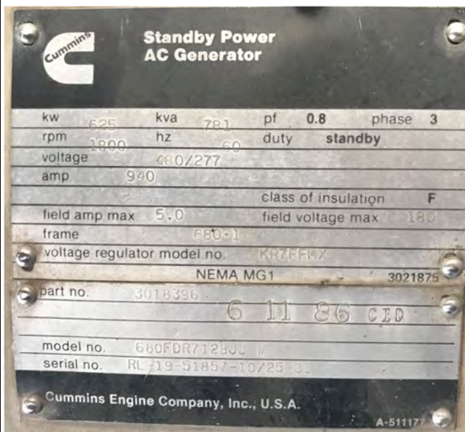
Figure 7-2 – Service 2 Generator Nameplate
